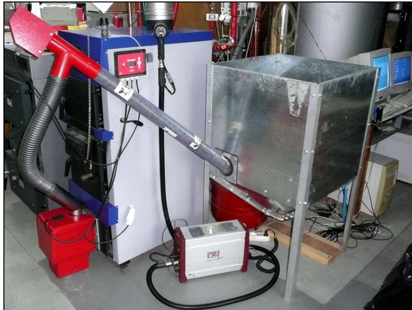
Fig.1. Heat station with two wood log boilers: with a heat output of 15 kW (with a pellet furnace) and 25 kW (with wood gasification)
